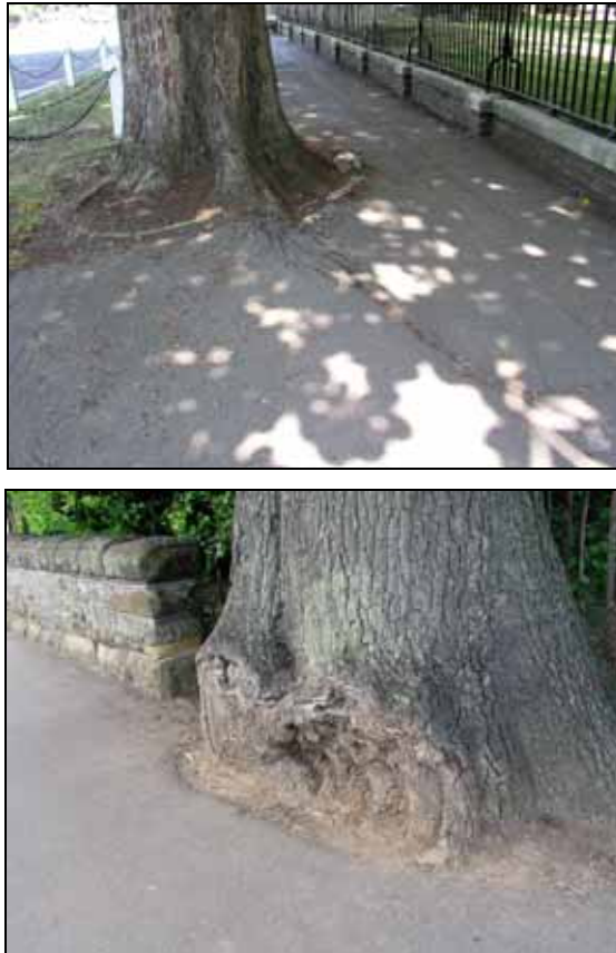
Figure 12 Examples of unsympathetic tree management: a) Tarmac laid right up to the bole of this tree has cracked and become unstable due to pressure exerted by underlying tree roots. In addition a cable has been laid very close to the trunk (right side) causing unknown damage to roots; b) This tree has clearly outgrown its location, and the lower part of the stem has been cut away to reduce encroachment onto the pavement. This damage could allow the entry of pathogenic fungi.
