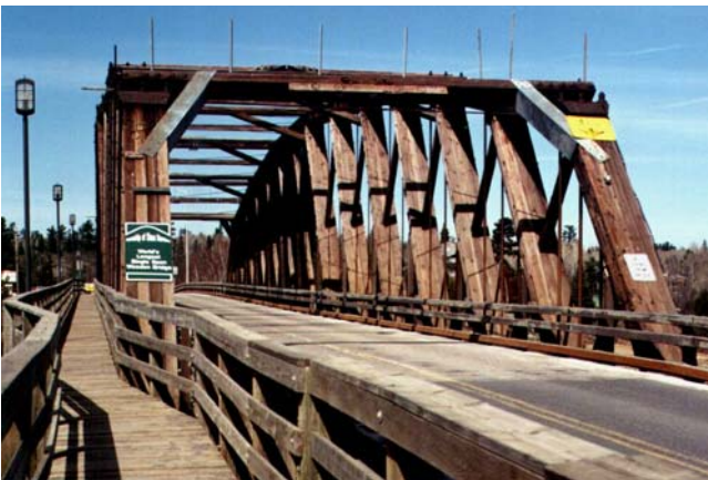
Figure 1 Sioux Narrows Bridge, Ontario, Canada built in 1936 (Photo courtesy of Ben J Haight)
