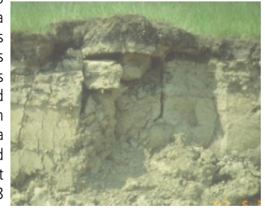
Figure 7. Damaged compacted clay cover system in southern Wisconsin caused by desiccation (Benson, 1999).
