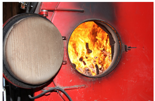
1610kw biomass boiler on the Witherslack Estate
