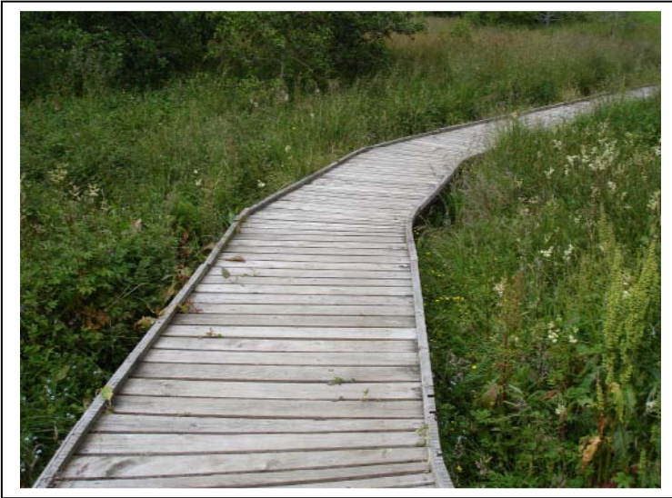
Edges to this boardwalk are good but the gaps between board are too far apart
