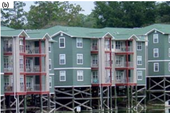
Figure 3: (a) 20-ton bearing capacity preservative-treated Southern Yellow Pine piles being installed for a lakeside residential development in Florida, USA (b) (photos courtesy of EW&S Contracting Co. Inc)
