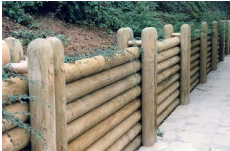
Figure 8: Roundwood retaining wall showing rounded ends to promote water run-off (photo courtesy of M&M Timber Ltd)
