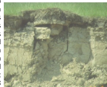
Figure 7. Damaged compacted clay cover system in southern Wisconsin caused by desiccation (Benson, 1999).
