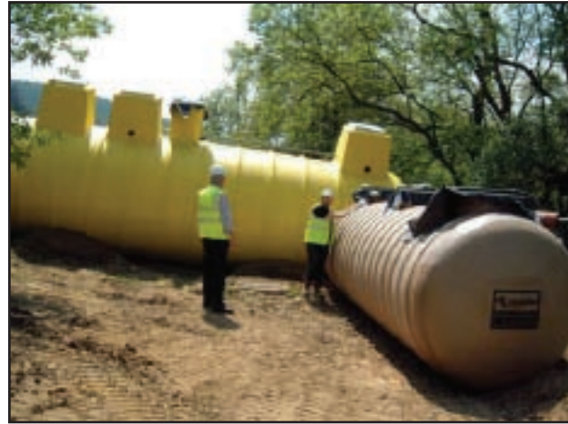
Sewage treatment tanks
