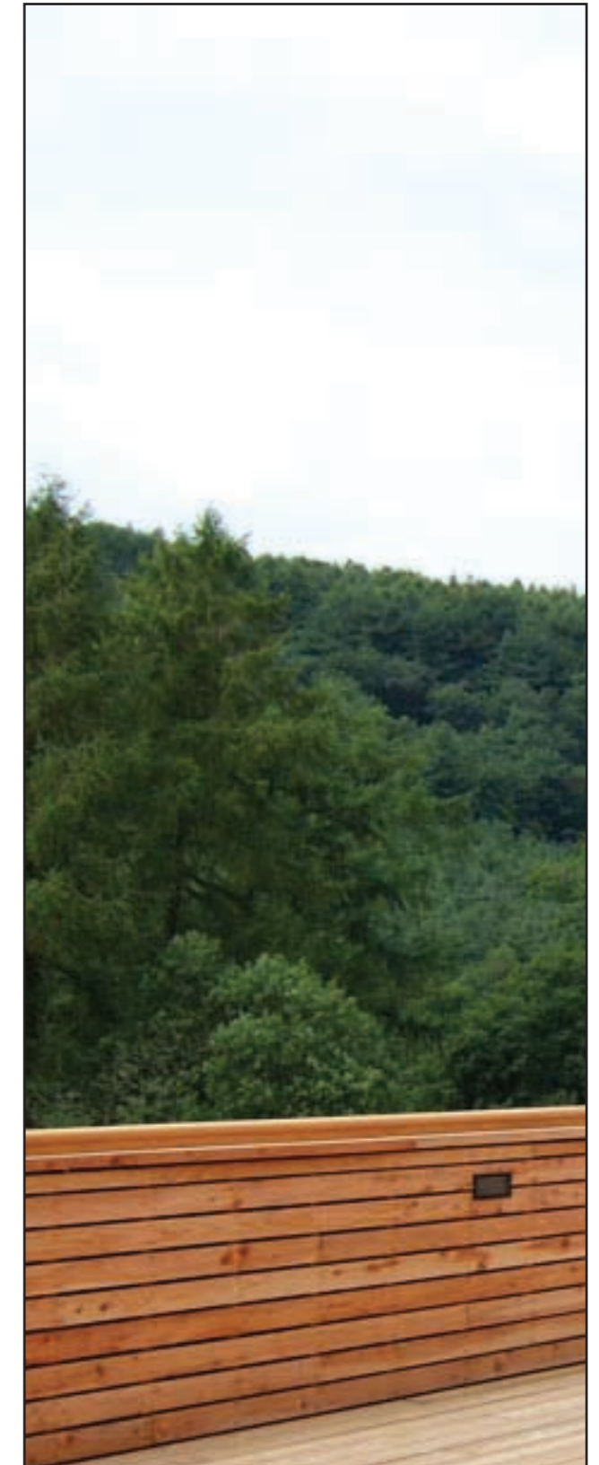
The building is clad in larch, grown and milled in the surrounding forest
