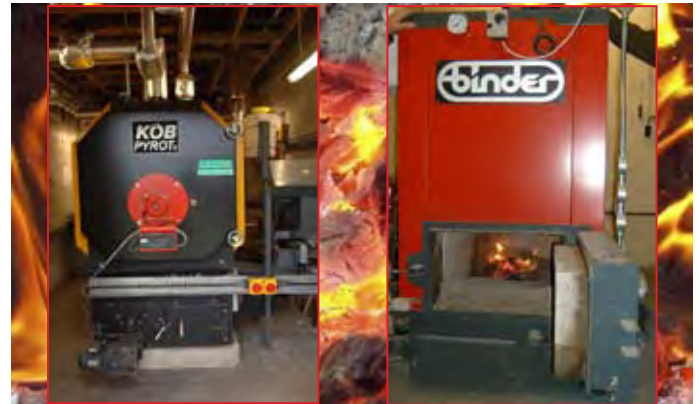
Woodfuel Boilers (photo: FC picture library)
