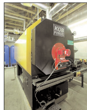
Inside the Kielder boiler house
