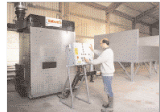
The Talbott’s B3 boiler and feed hopper
