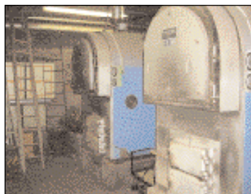
Converted boilers at Kirk Balk School
