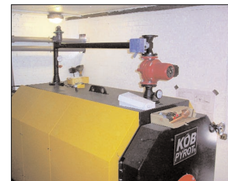
220 kW wood pellet boiler
