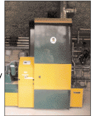
The KWB boiler system
