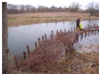
2. Laying down hazel brushwood to form a base on top of the deep sediment.
